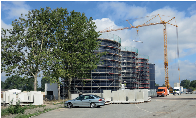
The biomethane production plant in Anklam.
